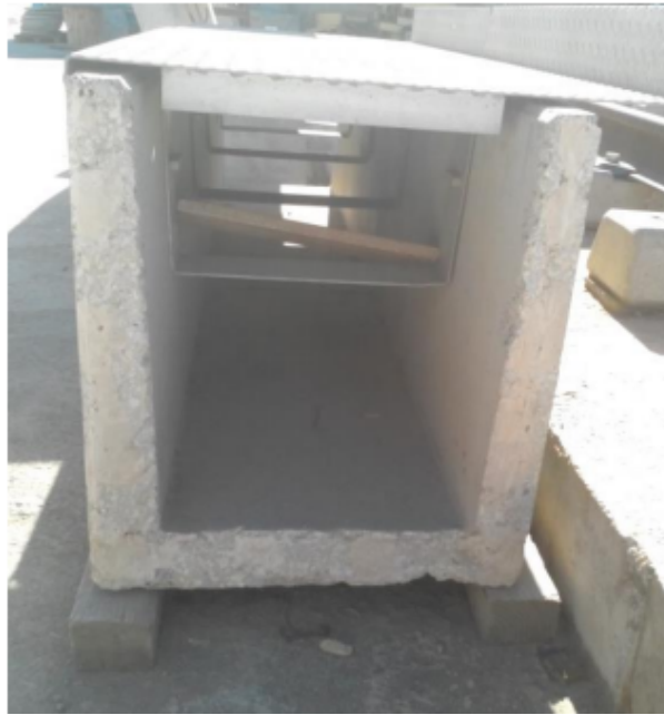
Figure 3.4: Cable trench of the existing line.
