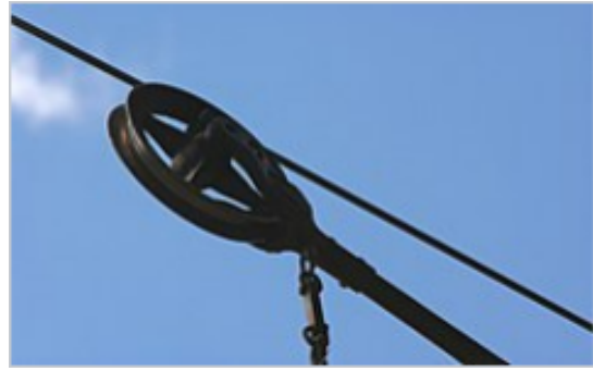
Figure 1.9: Trolley pole system.
