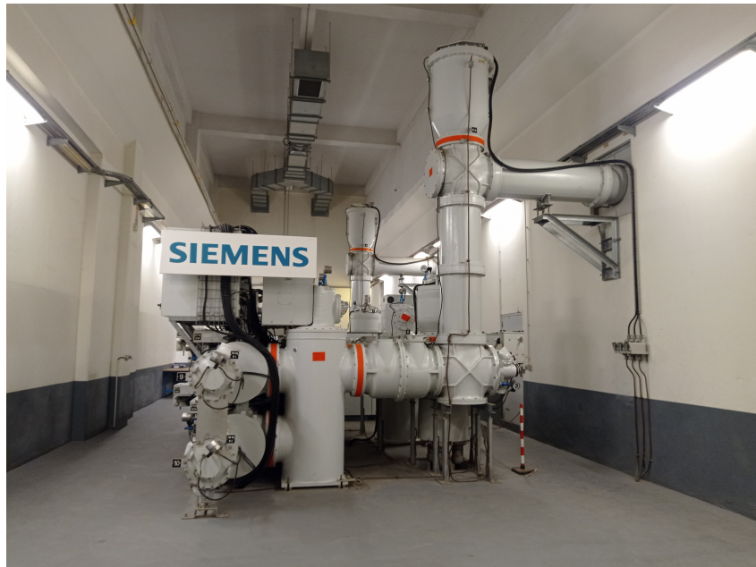
Figure 2.2: General view of the GIS
